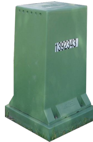
Electrical Distribution box
